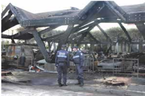
Burned garage in Suresnes, in the Hauts-de-Seine region.
